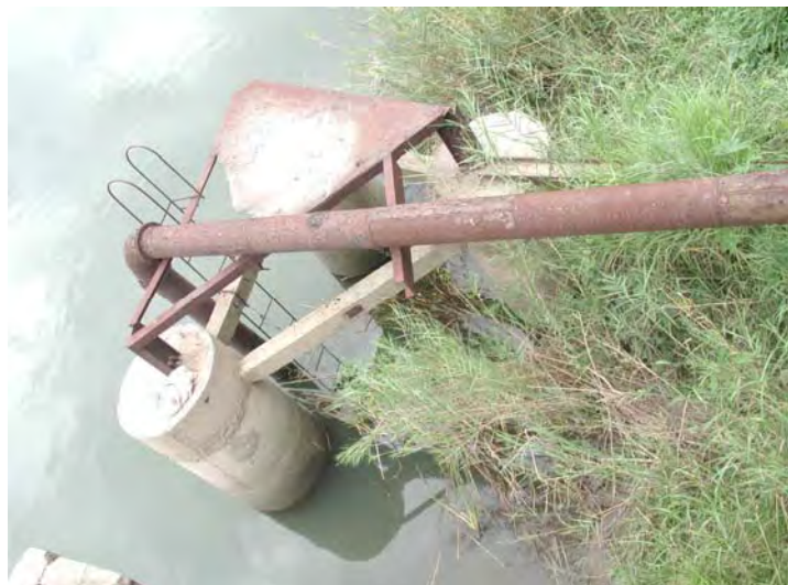
Magula pumping station's Water Intake
